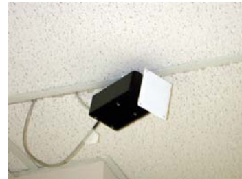
Figure 2. PAL650 UWB Receiver (Ceiling Mounted)
